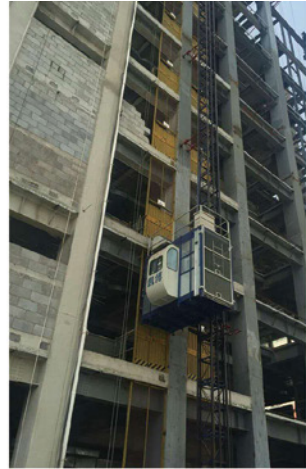
天津国贸240米变频调速升降机 Tianjin Guomao Building, VVVF building hoist (240m)
