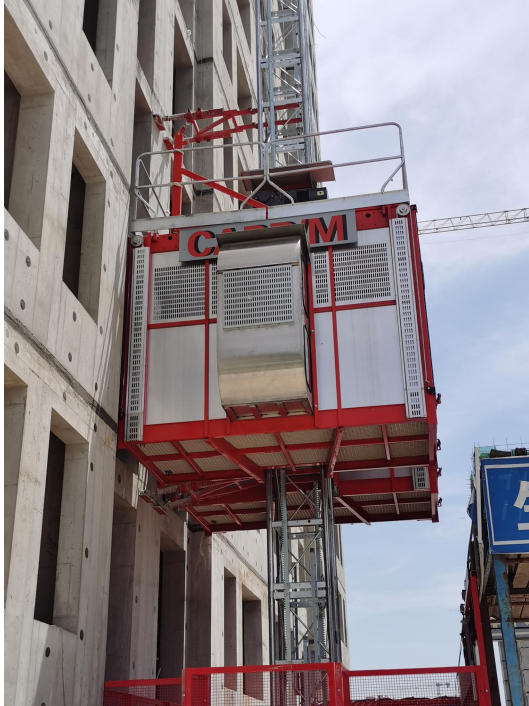
General building hoist
